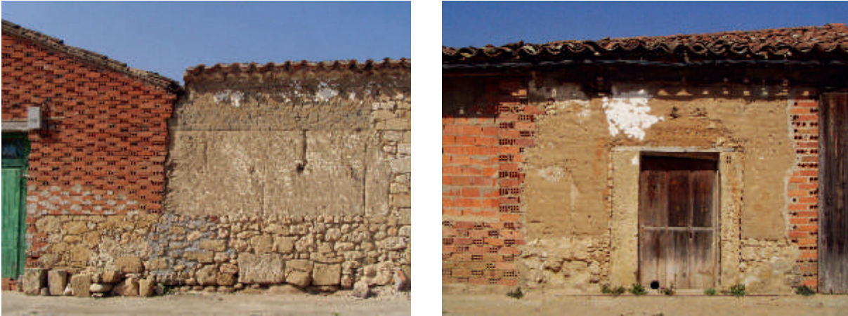
Fig. 2 Images showing the variety of techniques in vernacular earthen architecture. Home in Arcediano (Salamanca) with rammed earth walls built on ashlar foundation, crowned with adobe and repaired with hollow brick.
